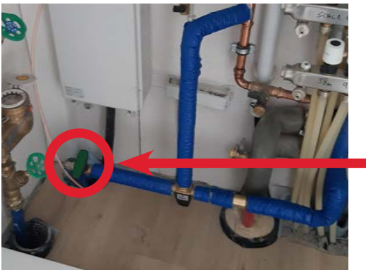
STEP 3: Open the cabinet in the entrance area (inside the house). Turn on the water tap (the tap may be located on the right) to fill the hot tub. (This takes approximately 35–40 minutes. Afterward, turn off the tap!)
